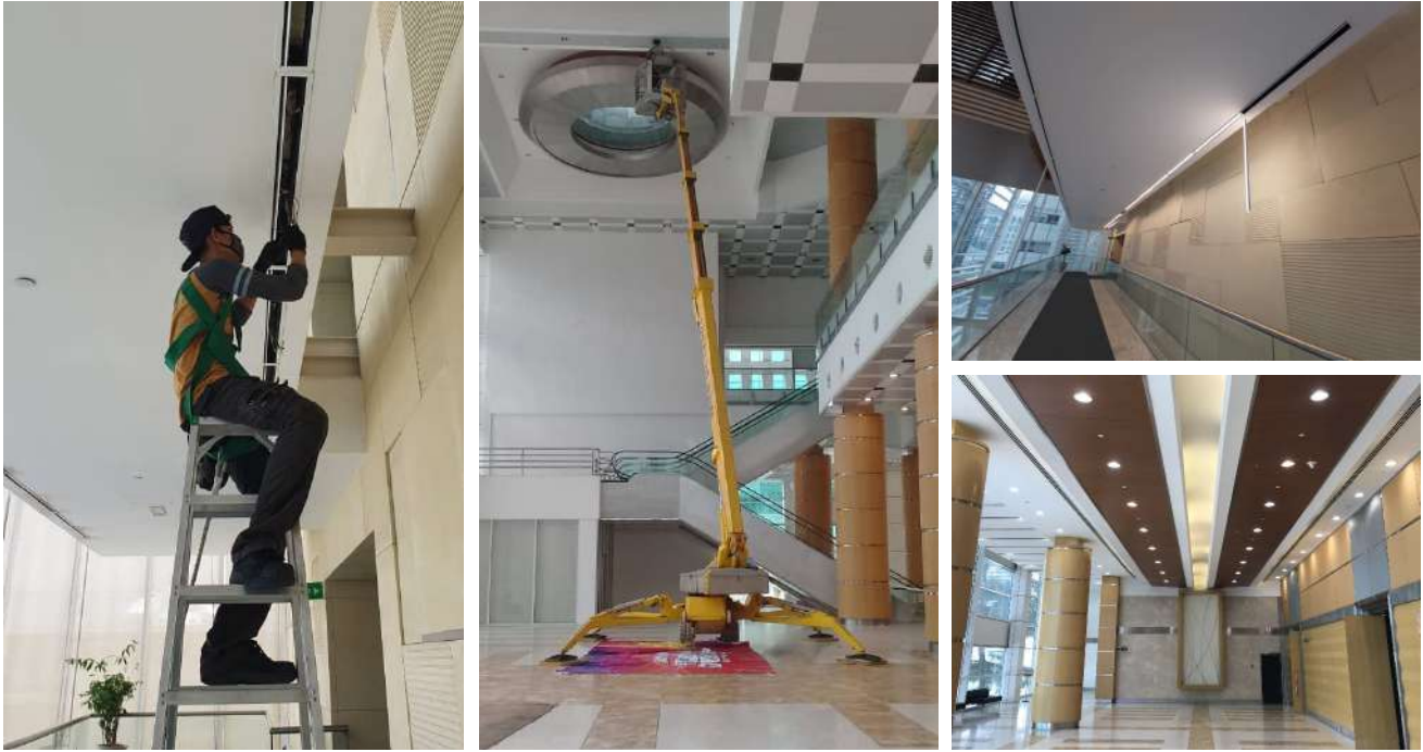
LED lights and motion sensors are fitted at office block corridors and hall's lobby area.
