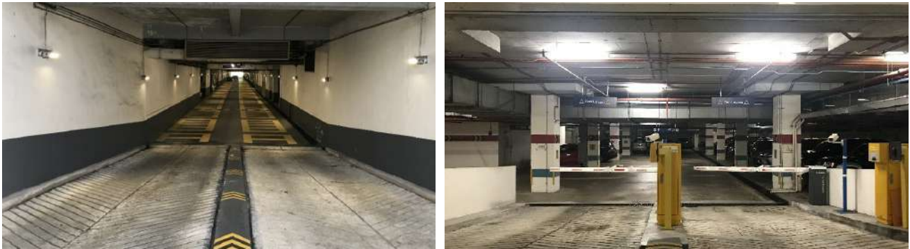
The parking areas have also been fitted with energy saving lamps (LED/T8) and motion sensors.
