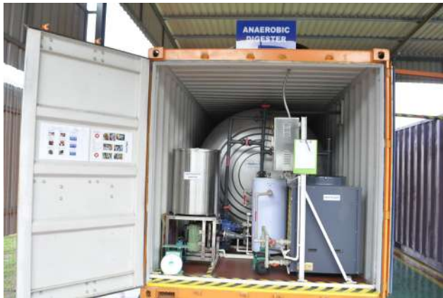
This AD machine with 500kg capacity can produce biogas and biofertilizers as a result of the food waste decompose process.
