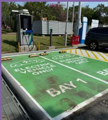
Charging stations (DC - 120kW) at Laman Perdana, Precinct 1.
