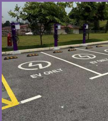
Charging stations (AC - 22kW) at Taman Saujana Hijau, Precinct 11
