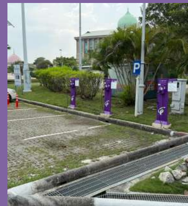
Charging stations (AC - 7kW) at Laman Perdana, Precinct 1
