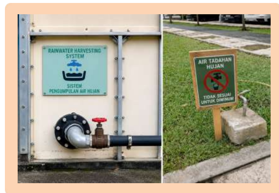
Rainwater harvesting systems
