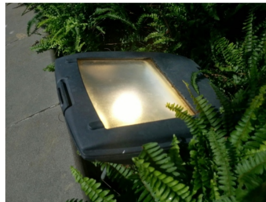
Lampu LED di courtyard, kompleks PPj
